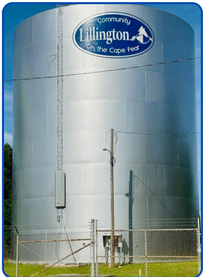
Town of Lillington ground-level water tank
